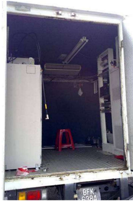
Figure 18. Interior of mobile BTS
