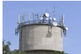
Figure 1b. Water tank
