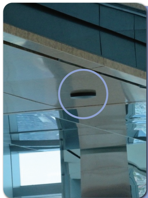
Picture 1: Access Point, Transmitter and Radio Communications Link inside The Exchange 106 Tower, Kuala Lumpur
