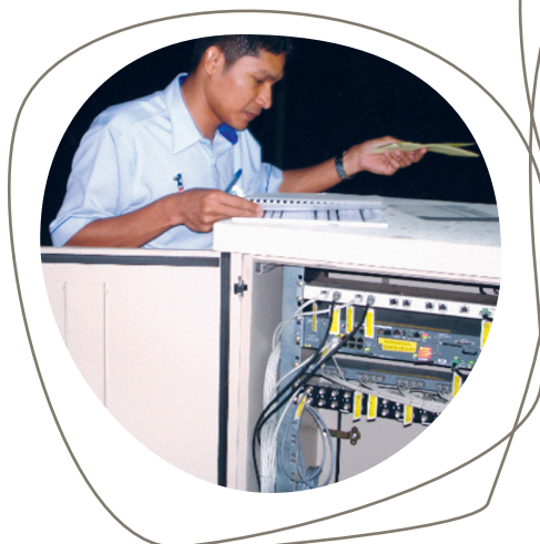
Apparatus Assignment inspection of a transmission station in Tuaran, Sabah.
