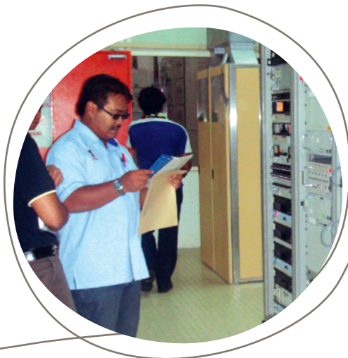
Apparatus Assignment inspection of a transmission station in Gunung Raya Langkawi, Kedah.
