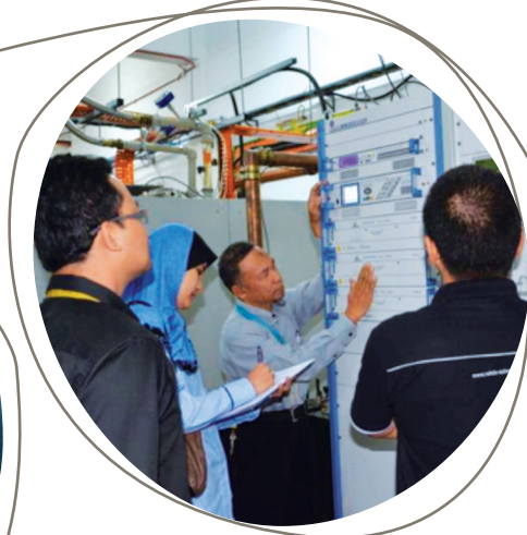
Inspection and verification of analogue TV trial transmission at TM Transmitter Station, Mount Kledang, Perak.
