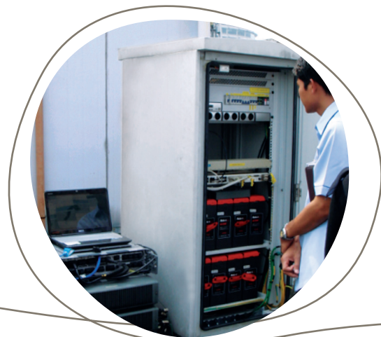
Inspection and verification of LTE trial conducted for Celcom Axiata Berhad at Bangunan Getah Asli, Kuala Lumpur
