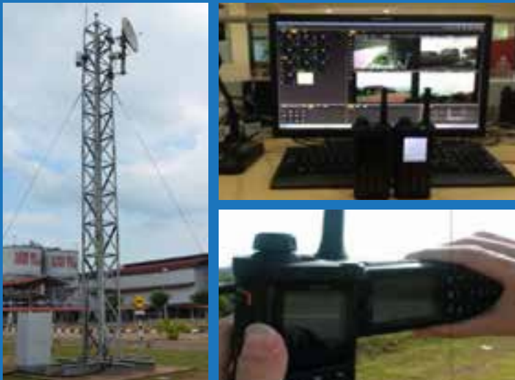
Photo: Inspection and verification on trial transmission for e-LTE at base station in Mill Sua Betong, Sime Darby Estate, Port Dickson, Negeri Sembilan.
