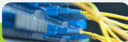
Communications Server (Encryption Enabled) (Category 5)
