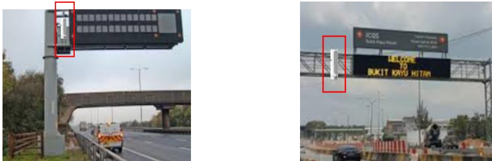
Examples of installation on gantry
