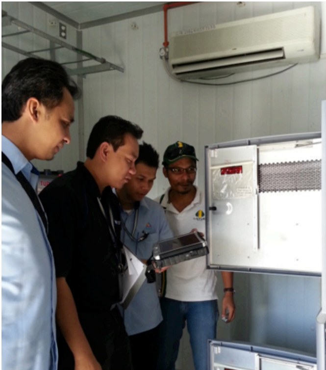
MCMC Officer inspect the transmitter station in Ulu Beranang, Negeri Sembilan
