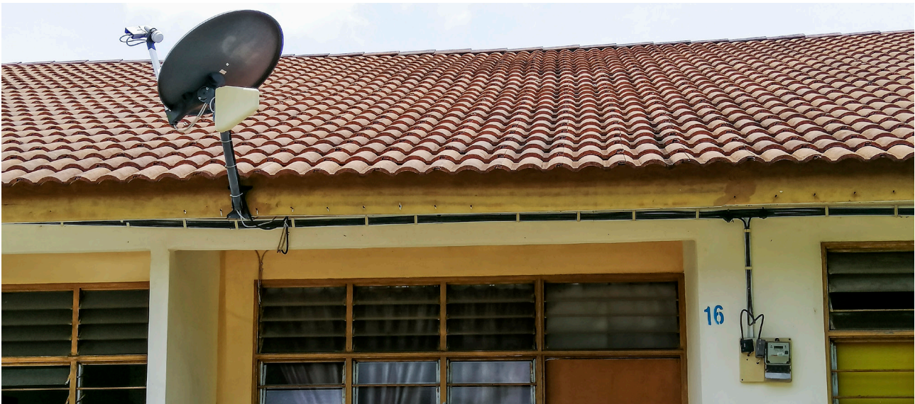
Cellular booster antenna
