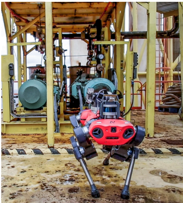
ANYmal robot used by PETRONAS in INSTEP, Terengganu to carry out monitoring activities on the oil rigs
