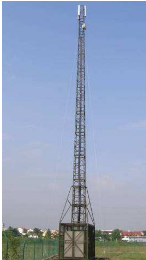
Figure 17. Portable BTS installation
