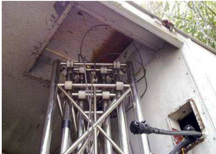
Figure 15. Rooftop opening to allow the mini-mast to extend through. The opening is for cabling infrastructure connecting antennas/microwave dish to the equipment.
