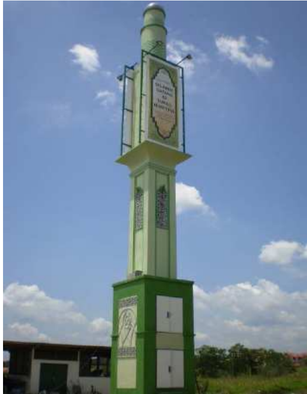
Figure 5. Minaret type (antenna come with integrated cabin) camouflaged by RF transparent materials to minimize visual impact.
