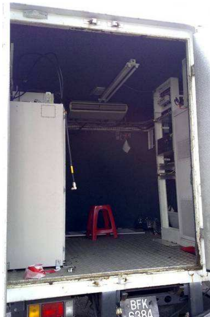
Figure 16. Interior shot of the cabin showing the BTS, rectifier and microwave racks. Also visible is the air-con blower.
